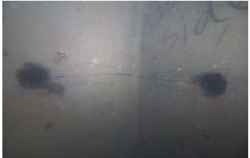
Damaged part of Water Ballast Tank No.7
